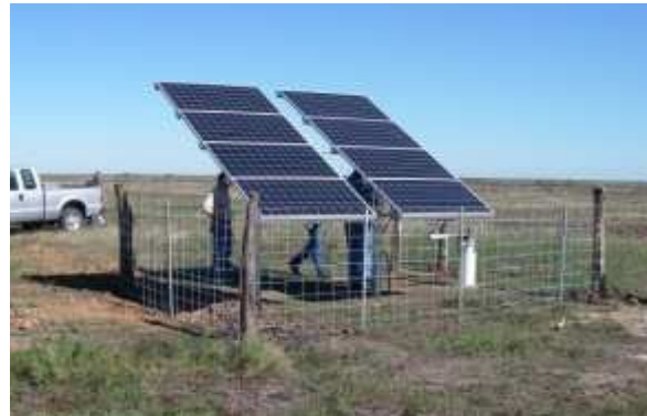
Small, solar-powered wells are ideal supplemental water projects for small wetlands (10 acres or less), as they ensure a constant water supply with few or no operating costs.
