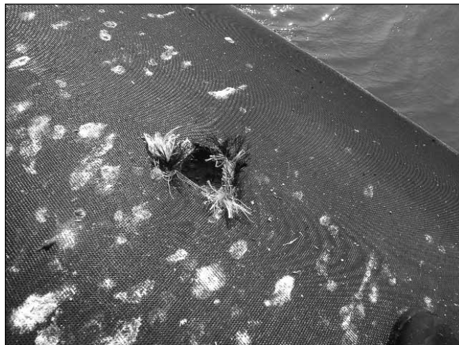
Intentional cut in the geo-textile breakwater.
