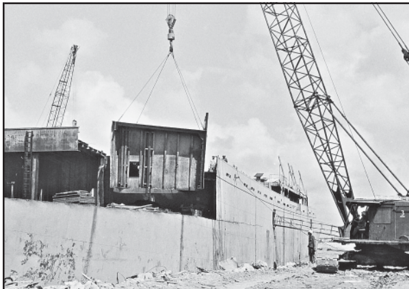
Figure 42. Sides were removed down to the last deck level (Texas Coastal and Marine Council 1975).
