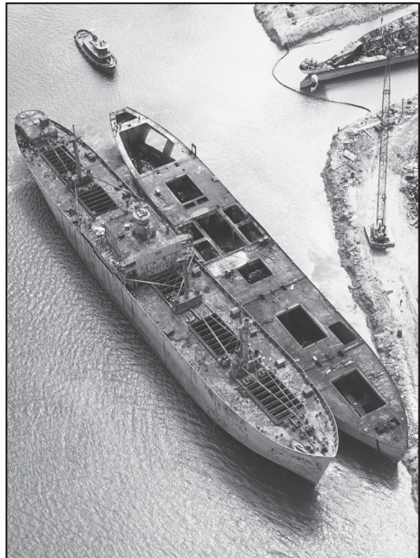
Figure 45. Aerial view of two of the twelve Liberty Ships that were prepared for sinking as artificial reefs. The ship on the right has had the superstructure and main deck removed. Deck openings seen here plus large side windows provide water circulation and access for fish (Texas Coastal and Marine Council 1975).
