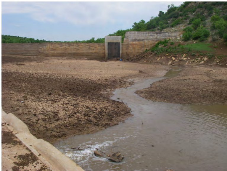
FIGURE 9. Muddy flat upstream of dam on Paint Creek, Haskell County, Texas, approximately 2 km below Lake Stamford Dam, May 2008.
