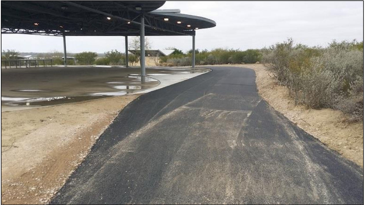
Photo showing access road constructed to and around large pavilion at Zapata County Boat Ramp Park. The access road will allow Largemouth Bass tournament organizers to use the pavilion and have drive-thru weigh-ins.
