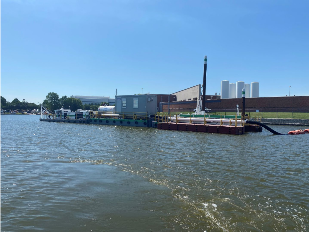
The dredging barge on Bachman Lake (May 2022). Photo posted by City of Dallas at https://bachmanlakedam.com/ .
